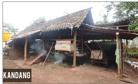
Photo 06 Separate cage with kitchen It is located behind the kitchen building Source : Personal Dokuments 2023
